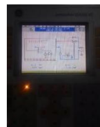
Gambar 4. Display Diane Genset Gas Engine [6]
