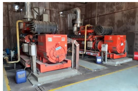
Gambar 7. Area Genset Pertamina Ep Asset 3 Tambun Field
