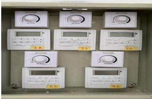
Gambar 3. 13 Panel Kontrol VSD
