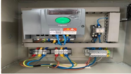
Gambar 3. 12 Panel Kontrol VSD
